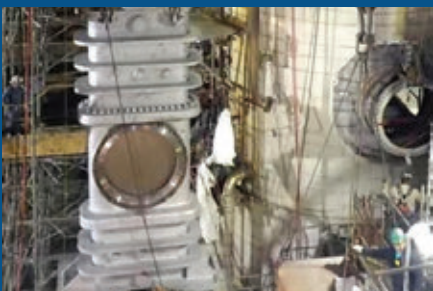
FCC Reactor Isolation
